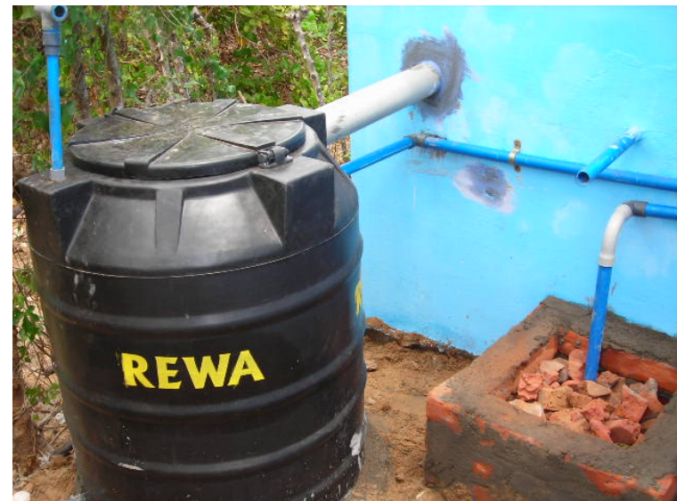
Urine collection tank and black water filter bed
