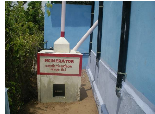
Incinerator, vent pipe and chambers
