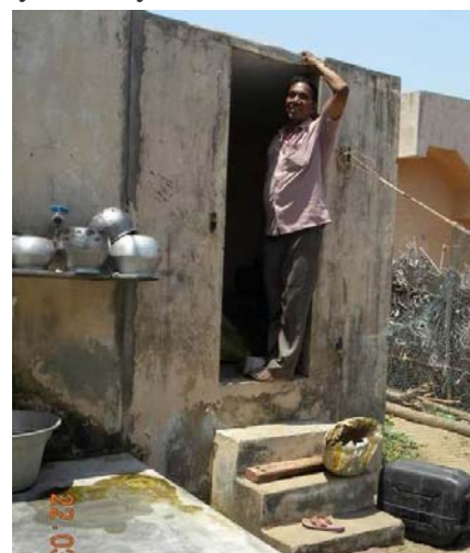
The roof leaky, too low and no doors for toilet
